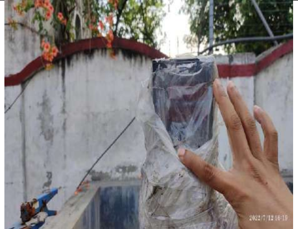
Pic.-17 Flowmeter at STP inlet (Flow-0.0 m 3 /hr)
