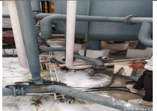
Photo 11: Filtration units installed in CPU
