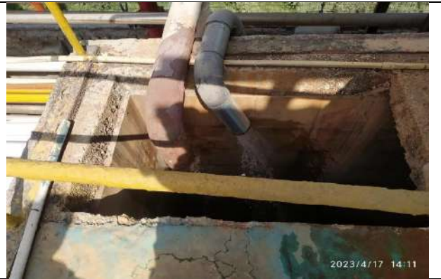
Photo 9: Inlet collection tank of CPU
