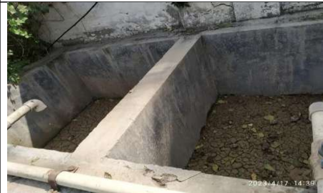
Photo 20: Sludge drying beds
