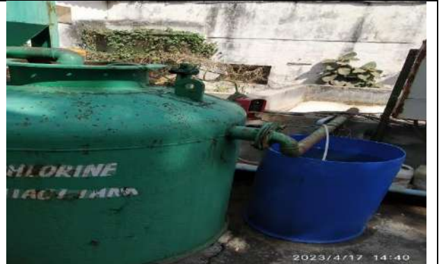
Photo 19: Chlorine contact tank and mechanical chlorine dosing system
