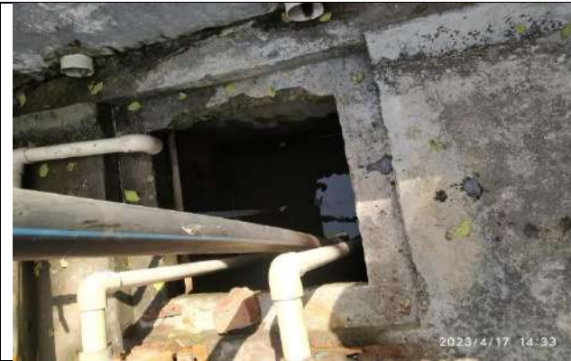
Photo 16: STP Inlet collection tank
