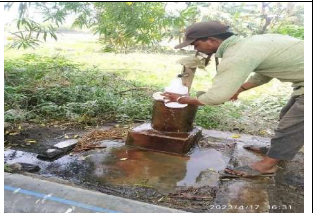
Photo 23: Handpump near compost yard at Ajeetpur
