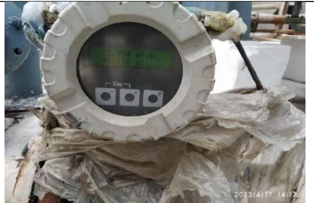
Photo 13: Flow meter at CPU outlet to cooling tower
