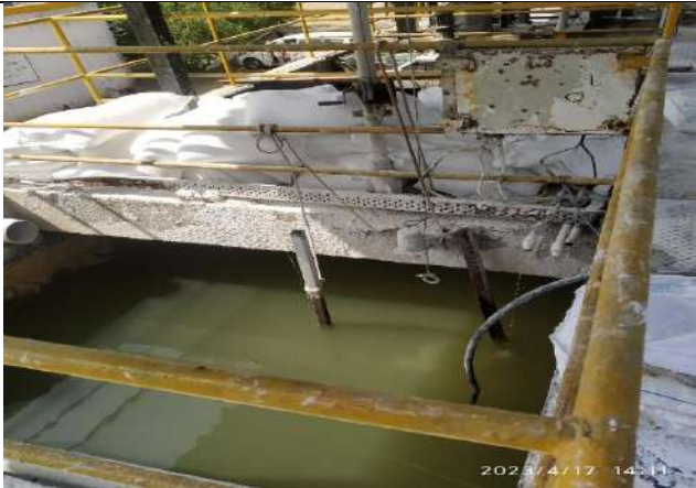
Photo 10: pH correction tank of CPU
