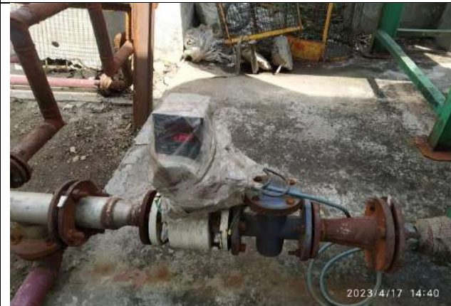
Photo 22: STP outlet flow meter
