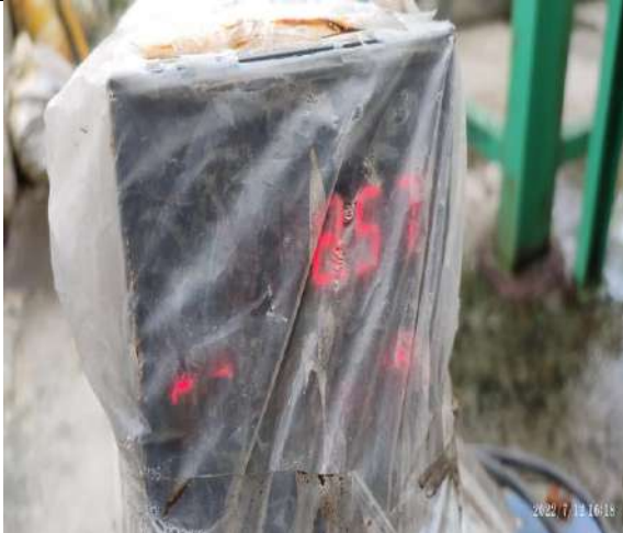
Pic.-16 Flowmeter at STP outlet (Flow-2.0 m 3 /hr)
