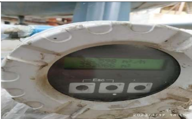
Photo 14: Flow meter at CPU outlet to Fermenter
