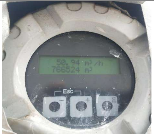
Pic.-19 Flowmeter at CPU inlet (Flow- 50.94 m³/hr, Totalizer- 766524 m³)
