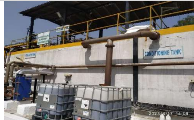
Photo 8: Condensate Polishing Unit (CPU)
