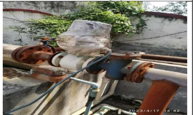
Photo 21: STP Inlet flow meter
