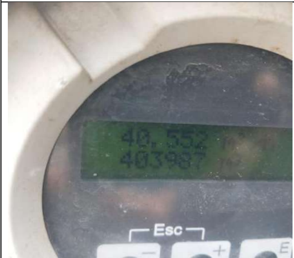
Pic.-20. Flowmeter at CPU outlet (Flow- 40.55 m³/hr, Totalizer- 403987 m³)
